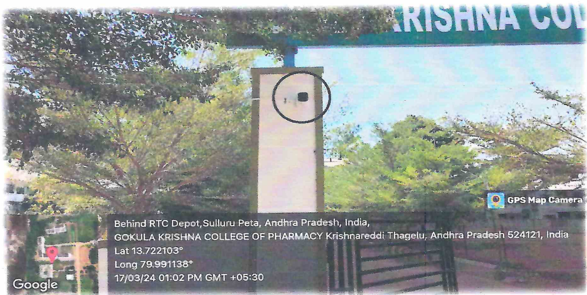
MAIN GATE CC SERVIVELANCE
